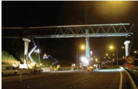
Above: With SH1 closed, Auckland Steel and NZ Strong undertake a night erection.
