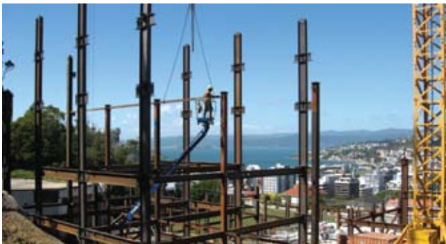
On an elevated and steep slope, erection proceeded quickly and safely at Victoria University Wellington.
