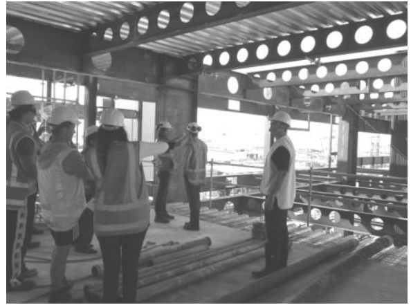
Students are briefed on the Britomart East project while work is in progress.
