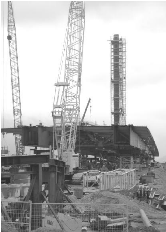
The Vancouver Coastal Meridian Over-bridge made of weathering steel, being prepared for launching.
