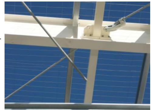
Rod bracing with failed connection
