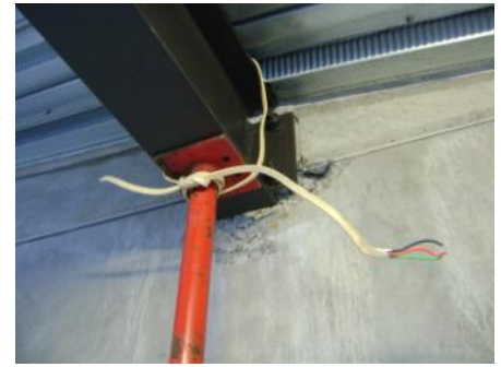
Spalling of cast in bolt connections
