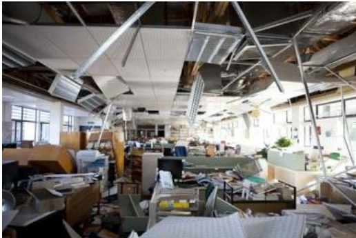
Non-structural damage at University of Canterbury
