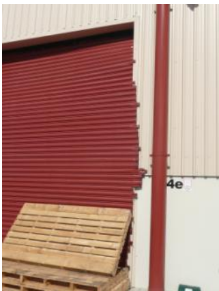
Damaged roller shutter doors
