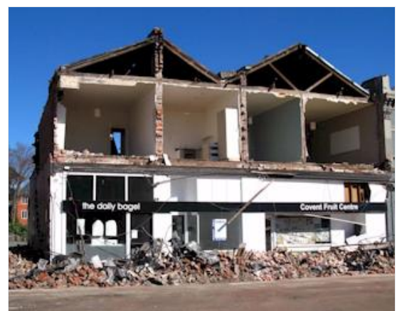
Wall collapse—unreinforced masonry building.
