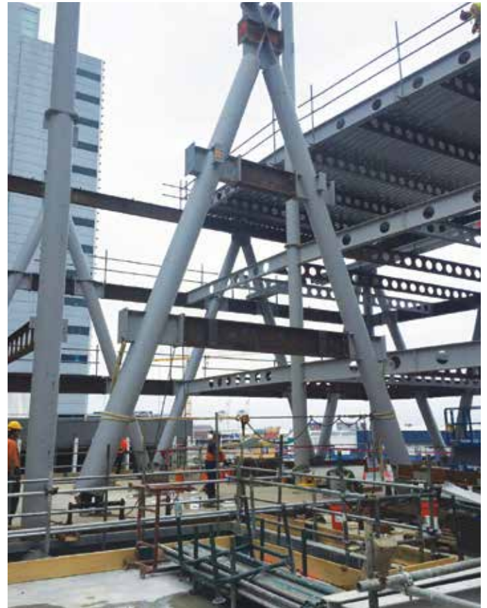
A-frame section of diagrid, upright and about to be released from a hinge frame and craned into position.
