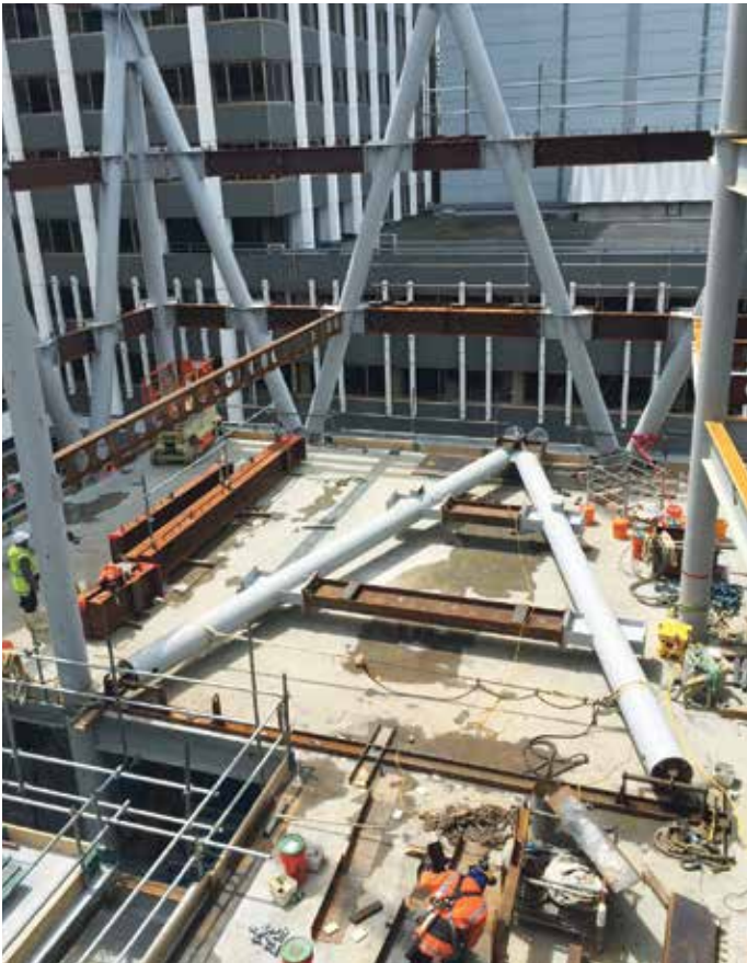
Diagrid A-frame section assembled on the slab in a hinge frame, ready to be lifted.
