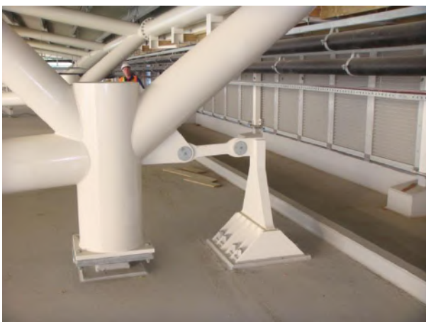
Figure 8: Energy dissipater restraining South Roof
