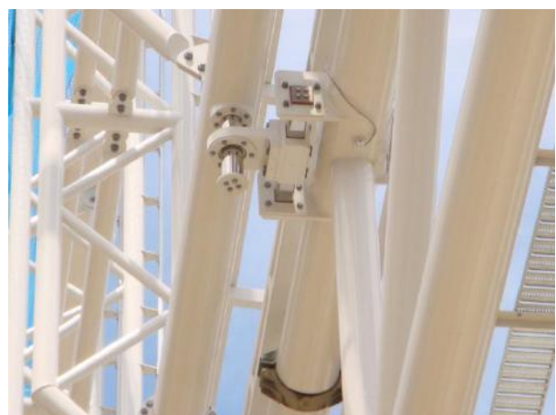
Figure 9: Two directional bearing between west hanging-facade and West Stand planar truss. Provides for vertical and longitudinal movement but lateral restraint.
