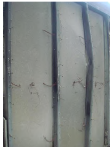
(b) After the fire test – Fire side
