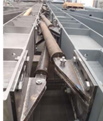
Figure 10: Mild steel fuse rods assembled with the braced frames in the workshop
