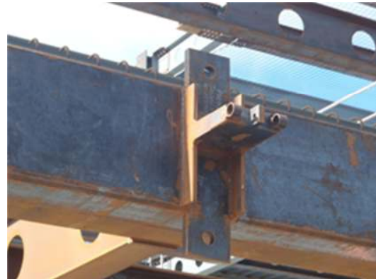
Figure 8: Tongue plate protruding from floor structure that slots through the seismic frame
