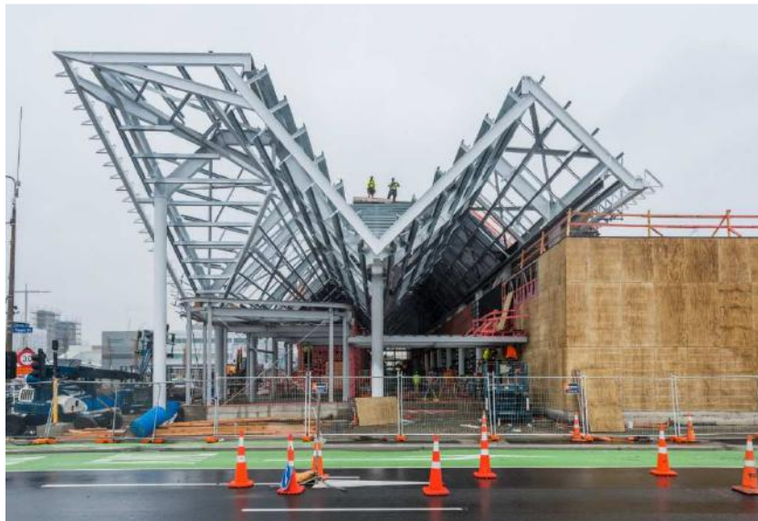
Figure 5: Image of the Christchurch Bus Interchange South Elevation under construction (image courtesy of Architectus)
