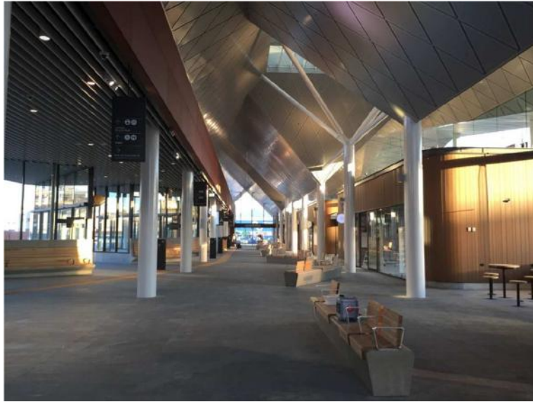
Figure 2: Image showing the Colombo building soffit which consists of folded aluminum panels on a secondary steel grillage (image courtesy of Architectus)
