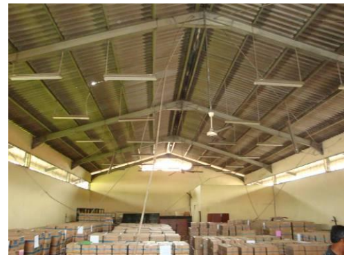
Figure 1: Collapsed Diagonal Rod Roof Bracing
