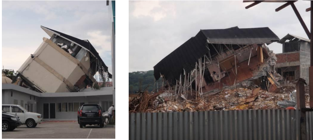
Figure 5: Collapsed Steel MRF with Partial Brick Infill Viewed From Each End
