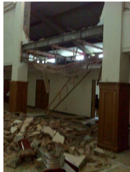
Figure 6: Collapsed Brick Infill Panel Above Public Area
