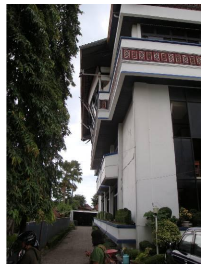
Figure 2: Wall Panel Separated from Roof
